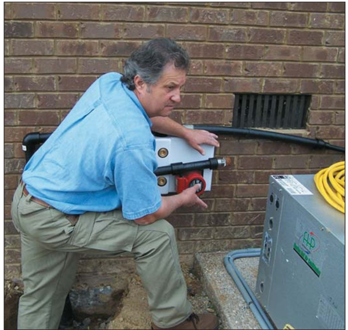
Sid Burks, owner of Sid Burks and Sons Heating and Air, inspects the geothermal unit installed in his son's home.
