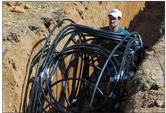
Brandon Burks installs underground coils through which a water-based solution will circulate. Heat will be transferred from the ground to the home and provide year-round comfort.
